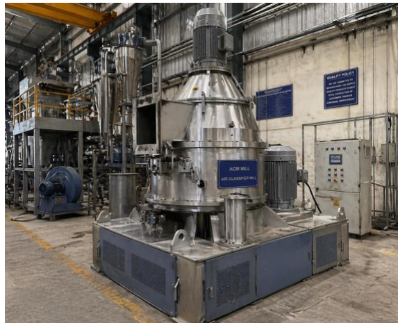
Figure 2 — Air classifier mill installed and commissioned
